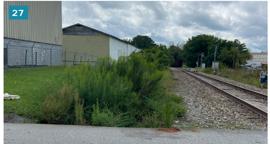
A ditch between the building supply and the rail line is a possible constraint.
