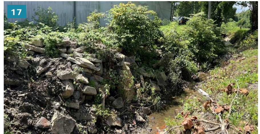
This unnamed tributary runs between several buildings, which limits a greenway connection between South Grove Street and parcels to the east.
