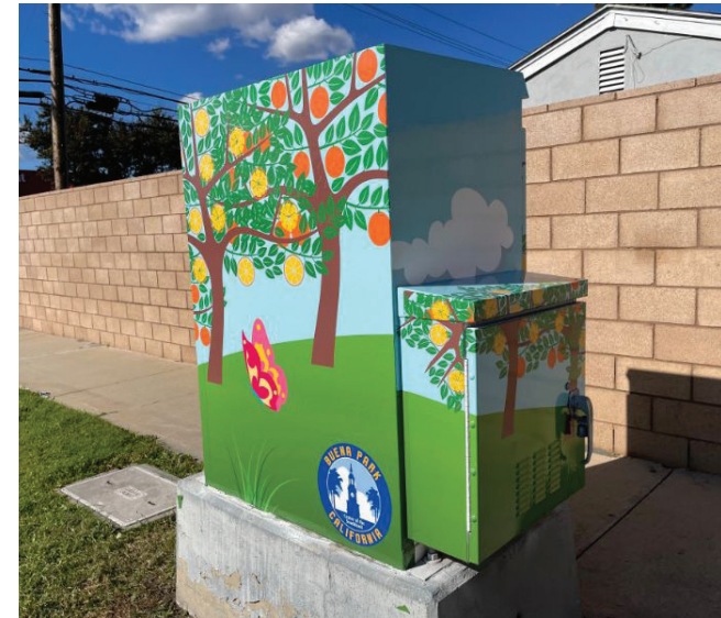
Electrical Box Vinyl Wrap in City of Buena Park | Superior Signs and Graphics
