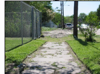
Examples of poor pavement quality
